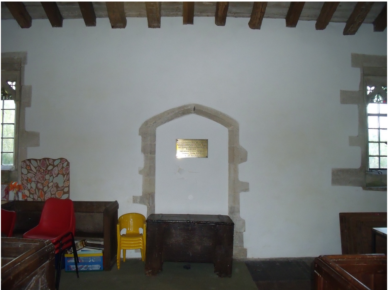
North Aisle – North wall – view from transept – as is – after December 2019 redecorate
